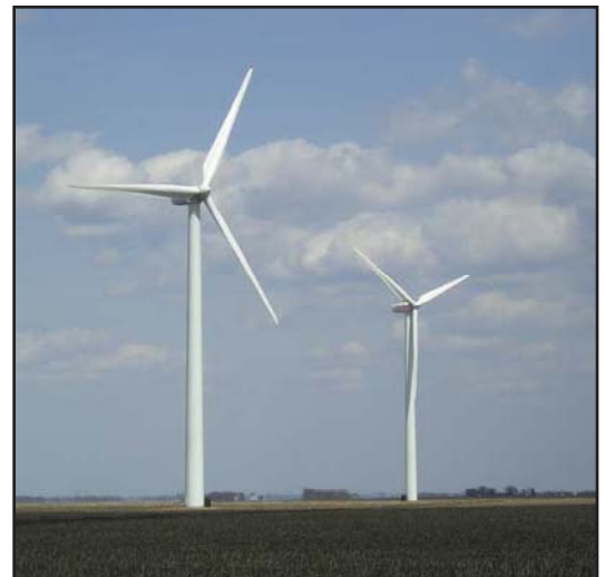
Figure 1: Three-bladed horizontal axis wind turbines.
