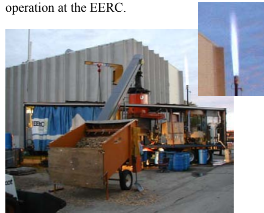
Figure 2 - 150 kW Portable Biomass Power Plant
