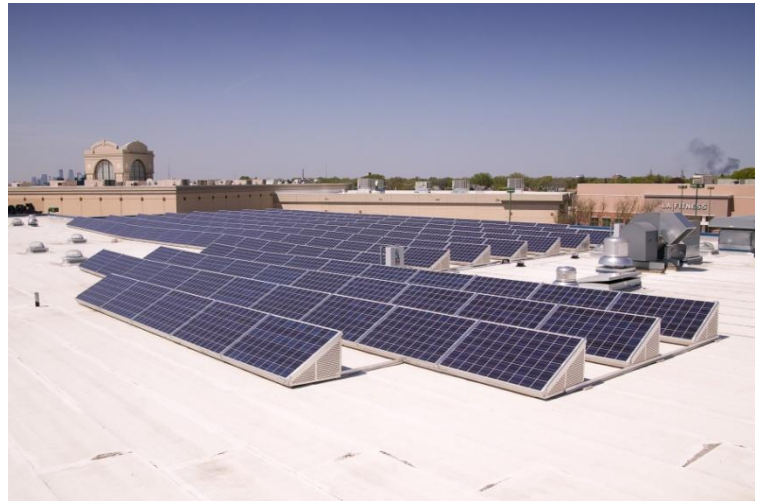
40-KW commercial PV installation on energy efficient white membrane roof, designed to fit around roof equipment to minimize shading (Western District Police Station, Saint Paul)
