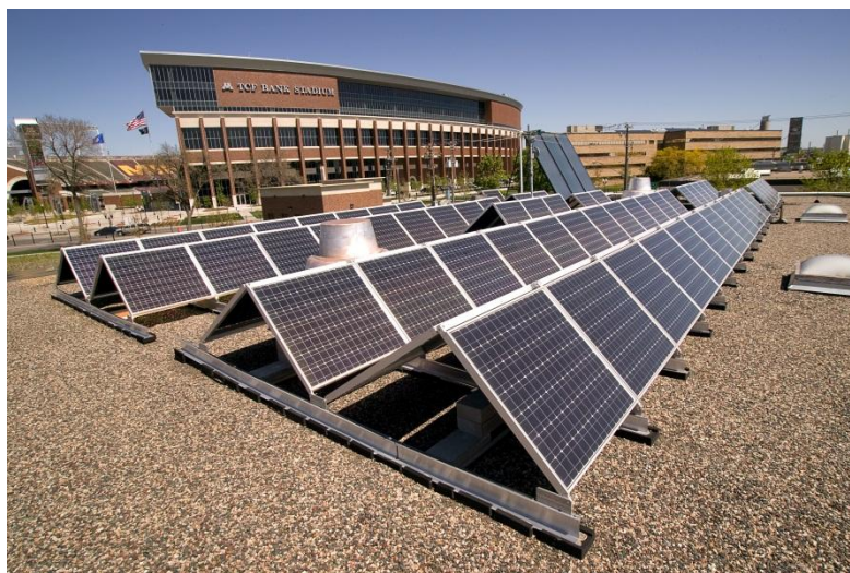
A 10-KW solar installation designed for a ballasted flat roof, with a solar thermal system in the far corner (Minneapolis Fire Station 19)
