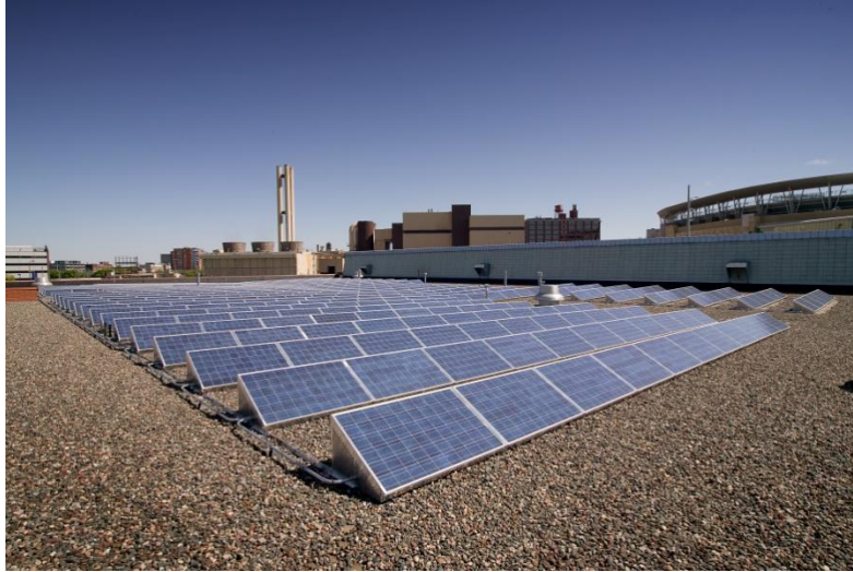
Roof space allowed for up to a 200-KW PV installation, but structural capacity limited the size of the installation to 40-KW on the Currie Maintenance Facility in Minneapolis
