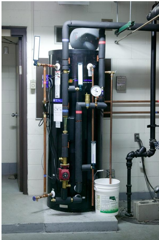
System design must integrate the solar installation into the building's mechanical systems
